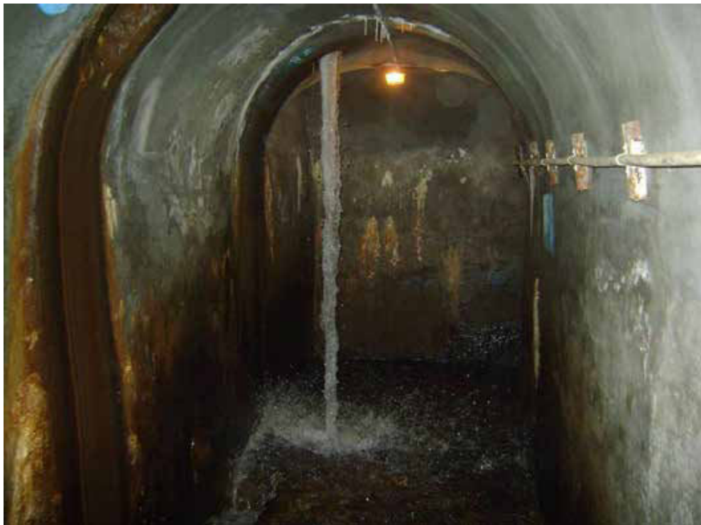
Picture 5 Ingress of the water into the drainage gallery by piping
